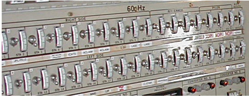
Figure 12. Panel with 34 switches.
